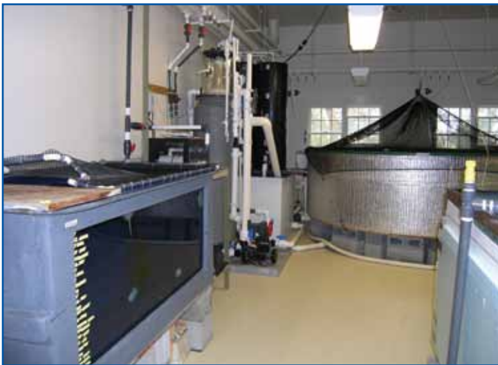
Behind-the-scenes tanks and life-support equipment used for supporting the skates and rays exhibit.
